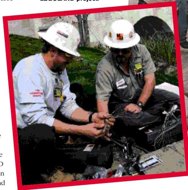
Below, Local 569 electricians Randy Loring (left) and Mike McComas install electrical controls for the LEGOLAND project.
