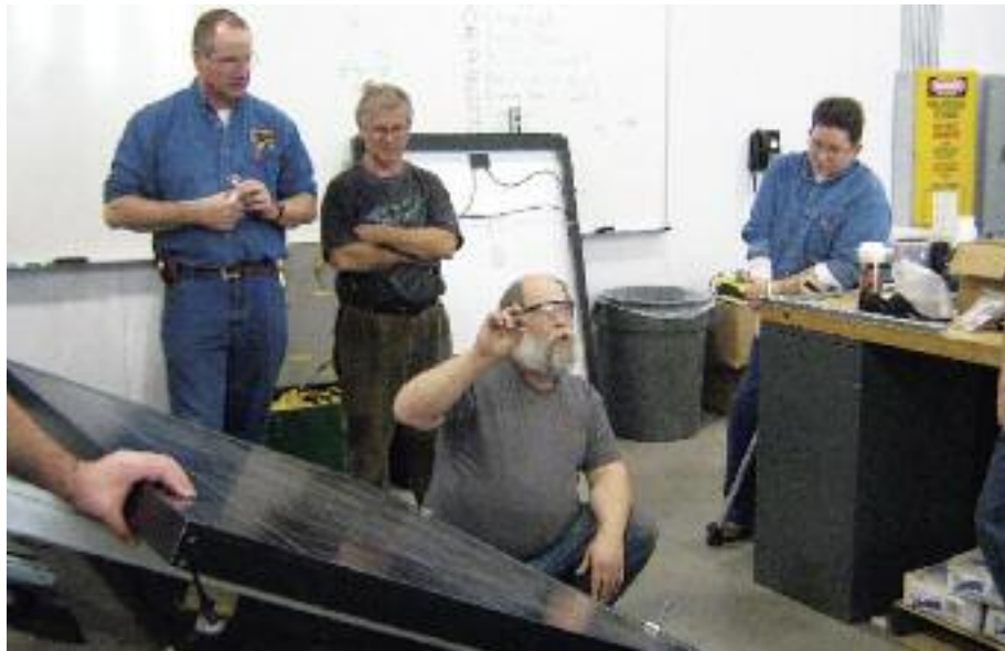
Minneapolis Local 292's JATC has a waiting list for members to train in solar installation. Veteran member Darryl Thayer, kneeling, instructs Bradley Kanis, left, Claude Clavette. Instructor Kelley Benyo stands at right.
