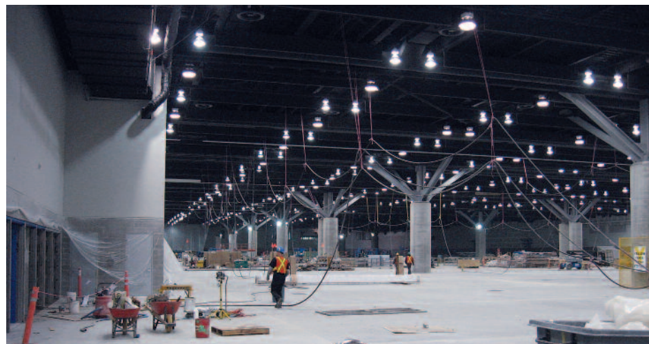
Vancouver's 1.2-million-square-foot trade and convention center will serve hundreds of thousands of visitors to the 2010 Winter Olympics. The center showcases the work of Local 213 members on a $36 million electrical contract for Western Pacific Enterprises.
