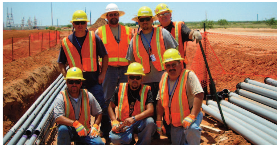
Albuquerque Local 611 members on the site of the $1.5 billion National Enrichment Facility in New Mexico. Clockwise from bottom center are Ralph Garcia, Pete Barrera, Brad McC Carson, Joseph Carl, Jonas Jaramillo, Ken Ziegler and Daniel Harbst.
