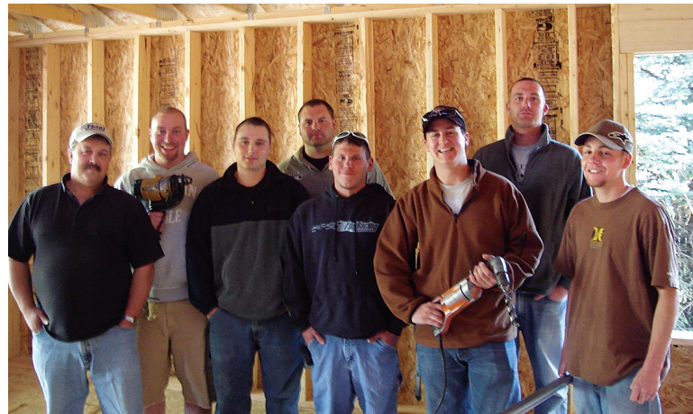
Members of Saginaw, Mich., Local 557 volunteer to wire a new house. From left are Apprenticeship Director Paul Dupuis Jr., Nick Zewerk, Joe Schmidt, Brandon Fink, Kevin Reinert, Bob Dupuis, Jason Reviette and Tom Haven.
