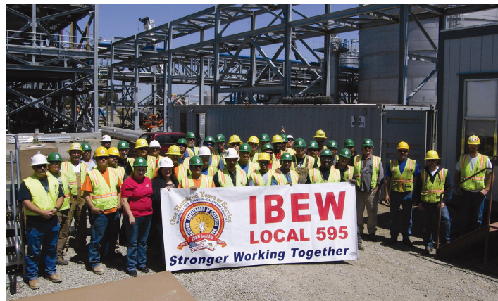
Over 50 IBEW Local 595 members are working on the Pacific Ethanol Plant in Stockton, CA, under a CURE-negotiated project labor agreement. The plant will produce 60 million gallons of ethanol annually when it comes online.
