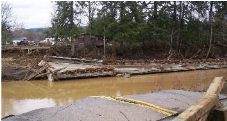
This bridge west of Adna, Wash., was destroyed by December mudslides.
