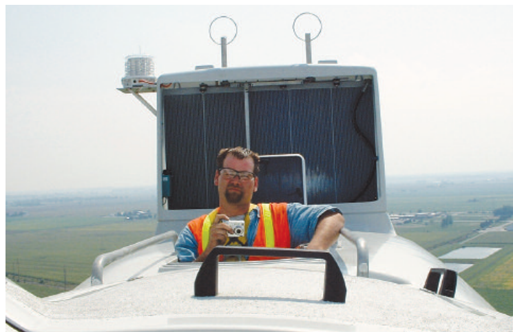
John Lock, Detroit Local 17 journeyman foreman at SPE Utility Contractors, stands atop a newly constructed wind turbine.
