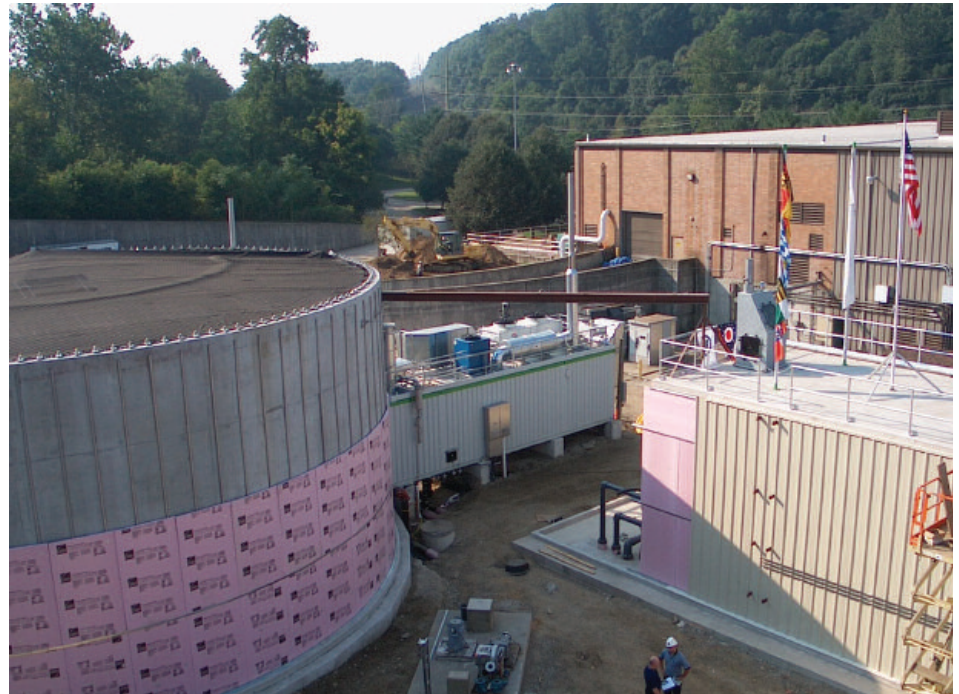
Akron Local 306 members helped turn an old compost plant into a wastewater-powered generating station.
