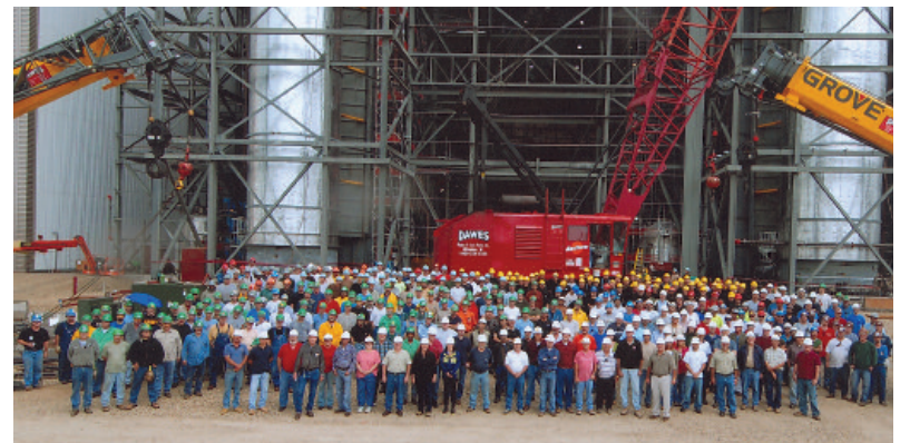
Milwaukee, WI, Local 494 members helped achieve a "2 Million Safe Hours" award for the Port Washington Generating Station.
