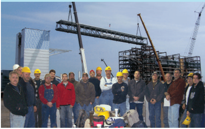
Local 56 members employed by Church & Murdock Electric Inc. at the Bayfront Convention Center. Cranes set the walkway bridge that spans the waterway connecting the hotel to the convention center.
