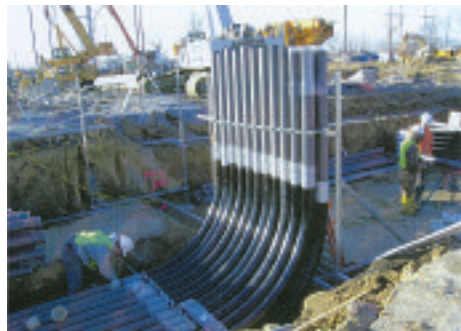
Local 193 journeyman wireman Neil Hervey ties down 5-inch pipe at the new Dallman 4 power station in Springfield, IL.
