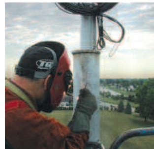
Local 58 member Tom Bowes welds pole together for the wind turbine at the training center.
