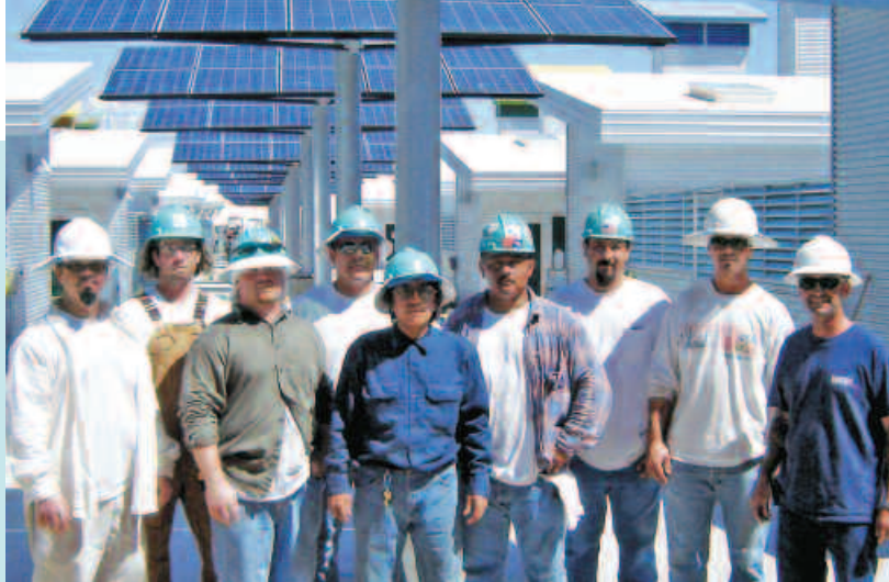
Las Vegas Local 357 members installed the solar array at the city's Regional Animal Campus, which was awarded a Nevada American Institute of Architect's Design Award last year. From left are Ramon Villalobos, Niles Mortenson, Travis Yourk, John Palumbo, Ed Samano, Robert Brooks, Santiago Rodriguez, Michael Andrieu and Chris Brooks, project manager.
