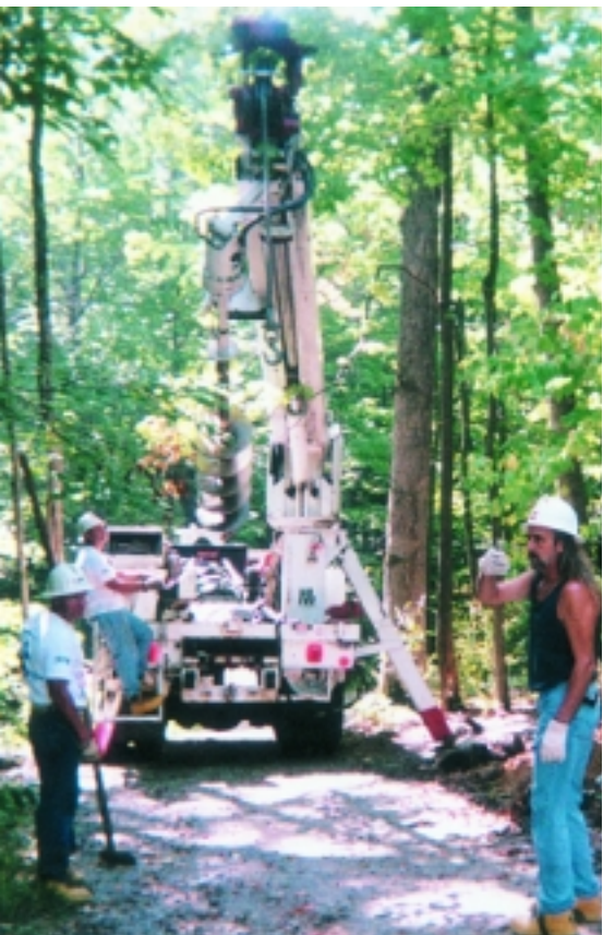
Local 1466 members working to make the electrical system safe at Girl Scout Camp Ken-Jockety in Ohio.
